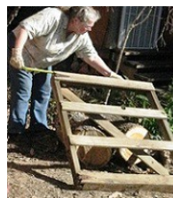
A not-so-narrow-gate: Kathy Young puts the finishing touches on the gate to replace the one that fell in the December rains
